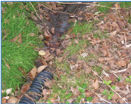
Suspected Illicit Discharge After inspection this connection was determined to be from a basement sump pump
